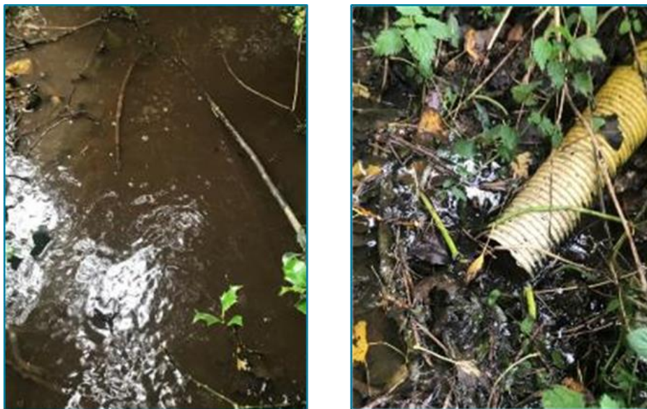
Plate 18.3.8: Silt Deposition and Outfall Pipe
