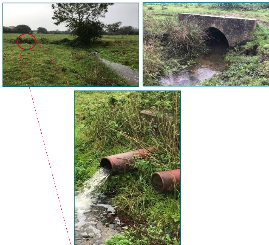
Plate 18.3.39: Outfall Pipes and Small Culvert
